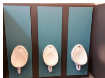
Urinals on service duct panels
