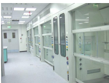
Walk In fume cupboards
