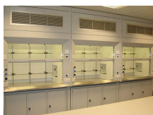
Re-circulation fume cupboard
